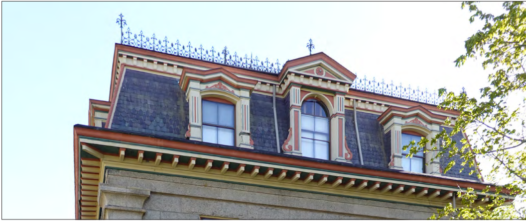
This slate, mansard roof includes three ornate dormer windows and a projecting wood eave. It is topped by delicate metal cresting.
