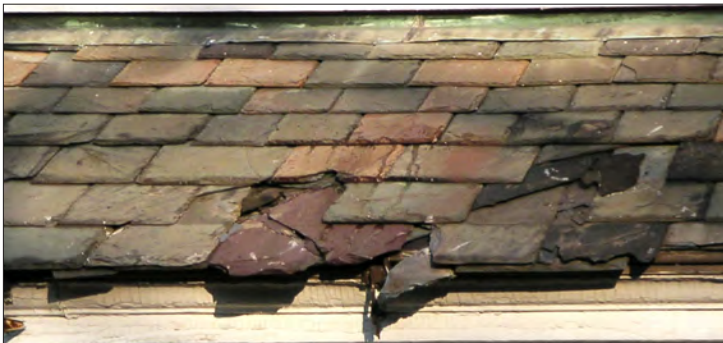
Missing or deteriorated roofing may allow storm water and snow melt to enter an attic, potentially rotting wood framing members. It is prudent to review a roof's surface as well as the underside of the roof where possible to quickly detect and repair roof leaks as soon as possible and minimize severe damage.
