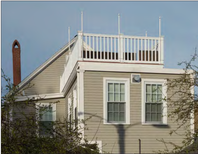
This roof deck, located on the rear wing of the house, is set back on one side and is minimally visible from the public way.
