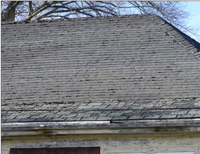
Deteriorated roofing can make a building highly vulnerable to water damage of the structure and interior finishes.
