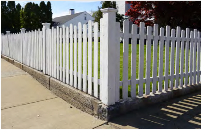
The details of wood picket fences can vary in detail. This example includes capped posts and rests on a masonry curb.
