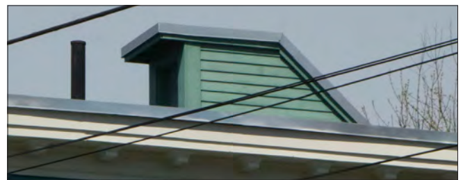
This penthouse houses a stair to provide access to the roof, with the size minimized by the sloped roof form. The penthouse is held away from the roof edge, minimizing its visibility from the public way.
