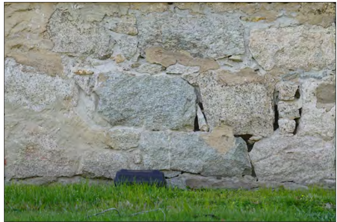
Mortar joint openings in stone foundations can provide a path for water and snow melt to enter a building as well as rodents and pests.
