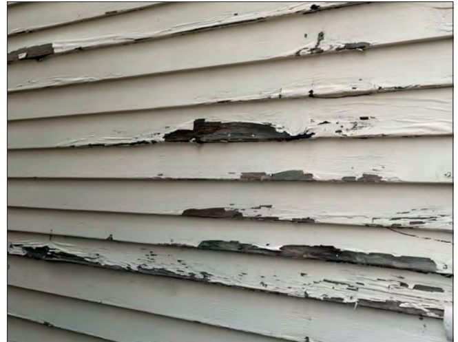
Exterior woodwork should be regularly repainted to reduce the potential for rot.
