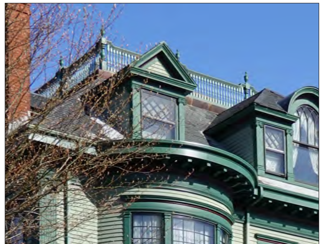
A widow's walk with a wood railing is located at the top of this roof.
