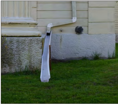
This downspout is painted to match the adjacent wall surface. The downspout extension directs storm water away from the building foundation.
