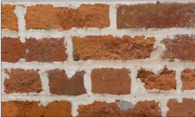
A saw was used to cut out the joints during repointing, thereby extending the vertical joints and damaging the bricks. In addition, both the vertical and horizontal joints have been widened.
