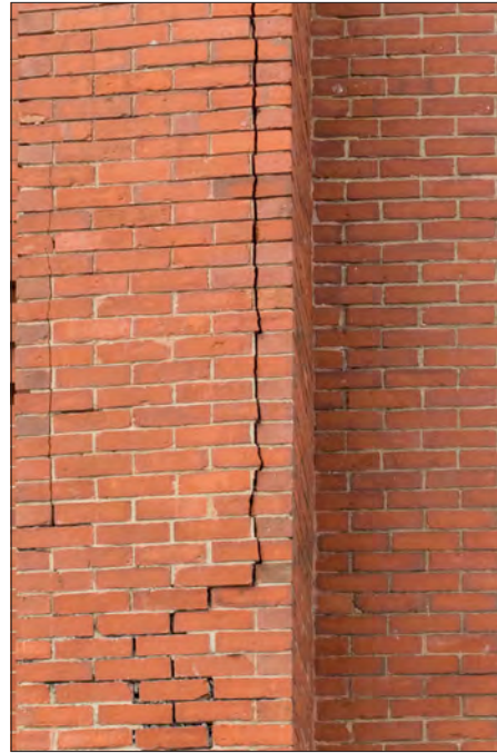
Long cracks at masonry, particularly cracks that split individual bricks or stones, can be an indication of a significant structural problem. In cases of more significant or recurrent cracking, consultation with an architect or structural engineer may be prudent prior to repointing.
