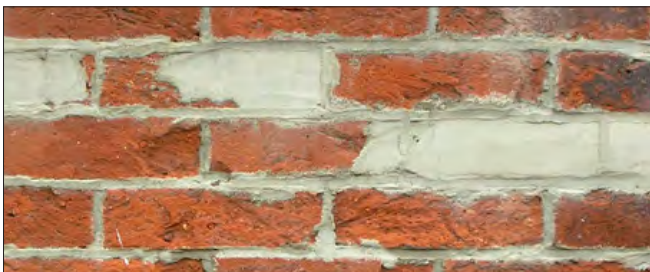
The rough texture and uneven surface suggest an aggressive cleaning method was used. Stucco patches replace bricks and efflorescence, a white powdery substance, can be seen on the surface.
