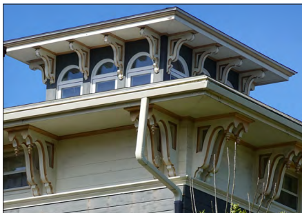
This cupola has a deep, projecting, bracketed eave similar to the one at the main roof, below.
