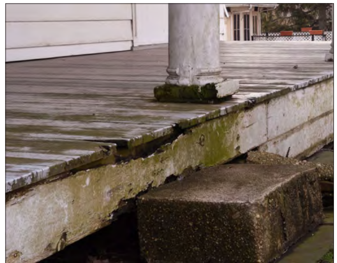
Porches, steps and other areas where the woodwork is laid horizontally or located close to the ground are often the first to deteriorate. Ongoing exposure to moisture can lead to rot of the column bases, porch deck and apron.
