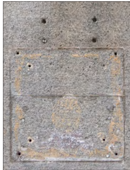
Numerous holes have been drilled into the face of this granite pier and several abandoned fasteners still remain. Fasteners should be removed, existing holes reused for future signs, abandoned holes filled and the stone surface cleaned. (Refer to Guidelines for Masonry and Stucco.)
