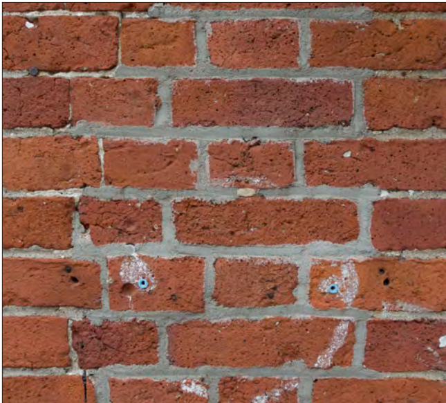
The central bricks have been repointed with what appears to be a Portland cement mortar that is harder than the hand-made brick. In addition, the mortar color and tooling poorly match the original mortar.
