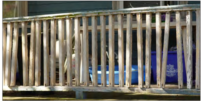
Loose elements of the railing should be re-secured.
