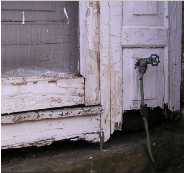
Leaking plumbing, including exterior hose bibs, can regularly expose woodwork to moisture, eventually resulting in rot. Wet wood can also be a desirable home for pests such as termites.
