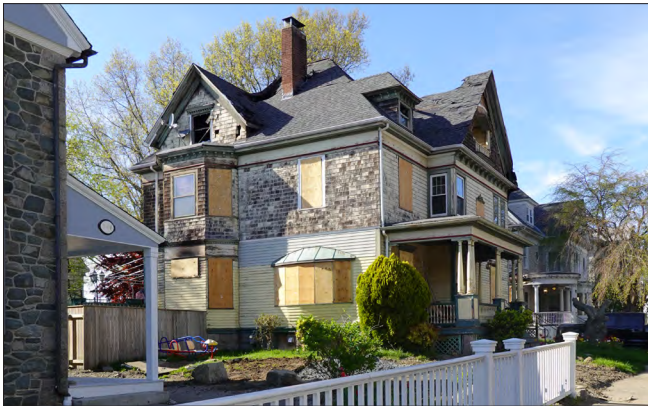
Sufficient information is available for this fire-damaged residence to accurately repair it and replace damaged elements in-kind.
