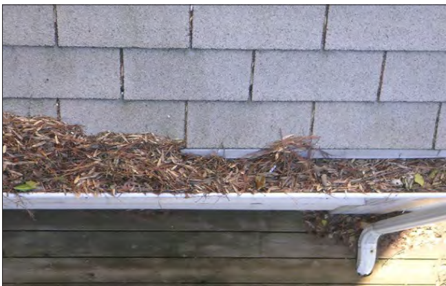
Regular cleaning of gutters and downspouts allows storm water to easily flow from a roof and away from building foundations, reducing moisture-related deterioration at wall surfaces.
